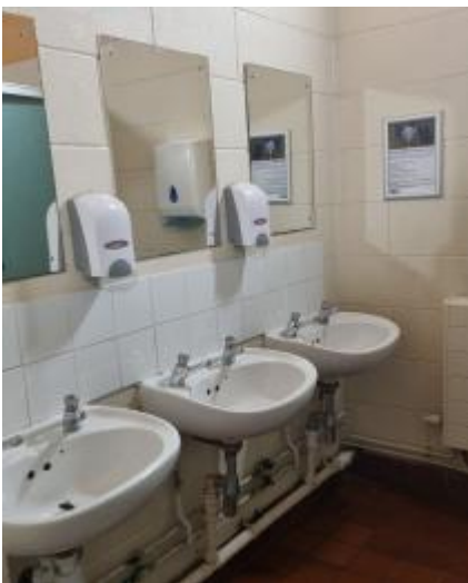
Sinks, mirrors and soap dispensers inside the toilets
