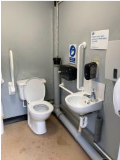
Visitor accessible toilet showing toilet and sink, plus grab handles
