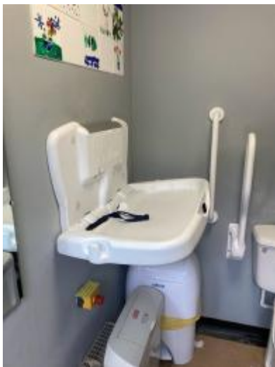
Baby change unit in accessible toilet
