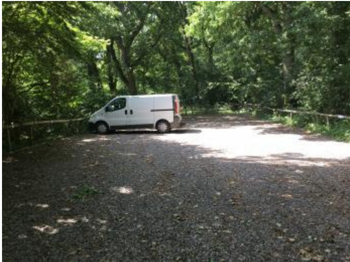
Car park rear extension. Loose and uneven gravel surface.
