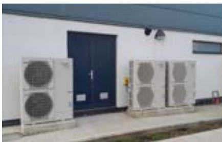
RSPB South Stack has replaced oil-fired heating with heat pumps – this minimises electricity consumption when moving away from fossil-fuel heating systems
